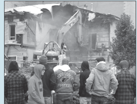
Construction trades students from R.G. Drage Career Technical Center, under the supervision of instructor Brad Richardson, helped the Museum prepare for the groundbreaking ceremony, then they returned to watch the demolition of the Knox Building. MV
